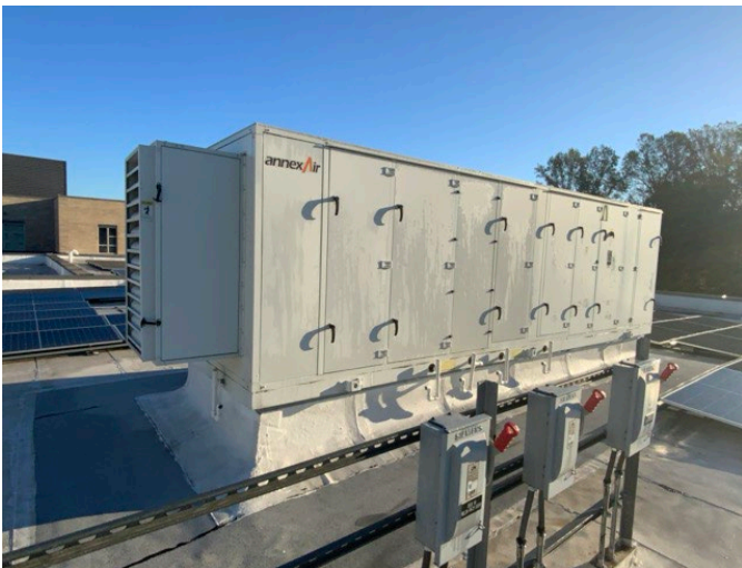
27 - ENERGY RECOVERY UNIT
